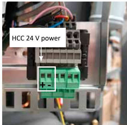
②b B2 - HCC terminal block - Internal unit signal
