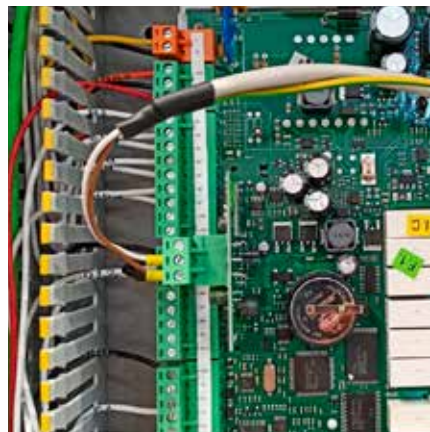
⑦b μPC BMS connection
