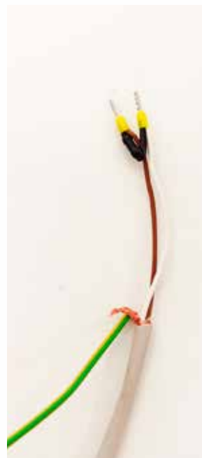
③ Green/yellow shield ground connection
